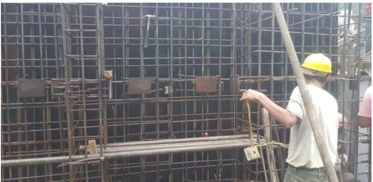
Figure 5.6: Installation of first stage embedded parts at undersluice gate and stoplog groove.
