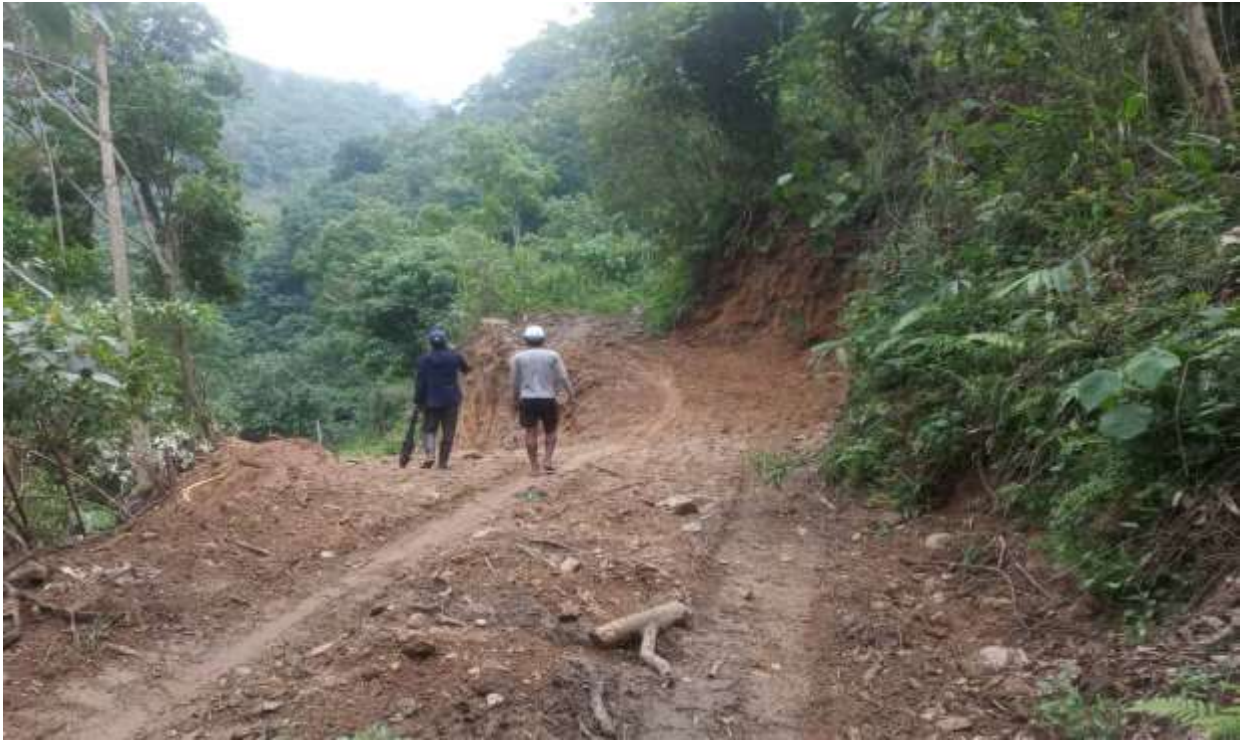
Figure 5.16: Excess road from powerhouse to surge tank.
